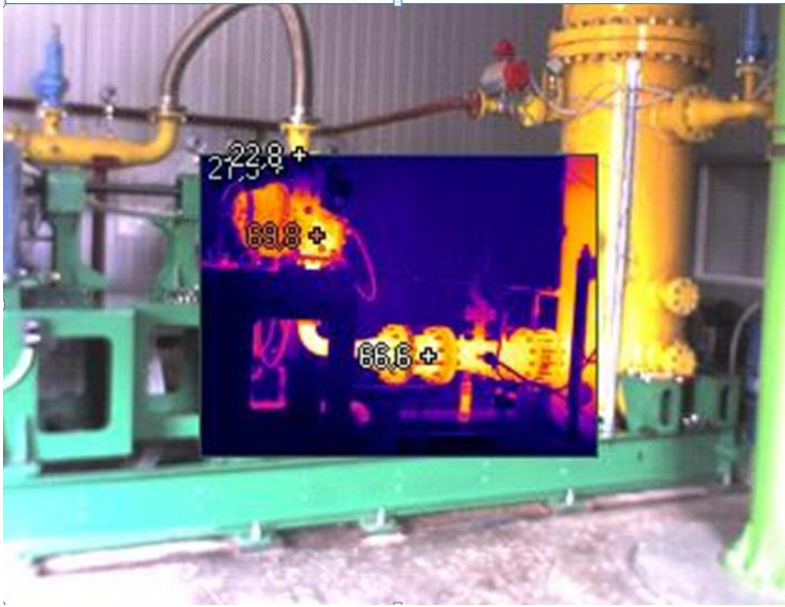
Fig.7- Temperatures of the compressor surfaces
