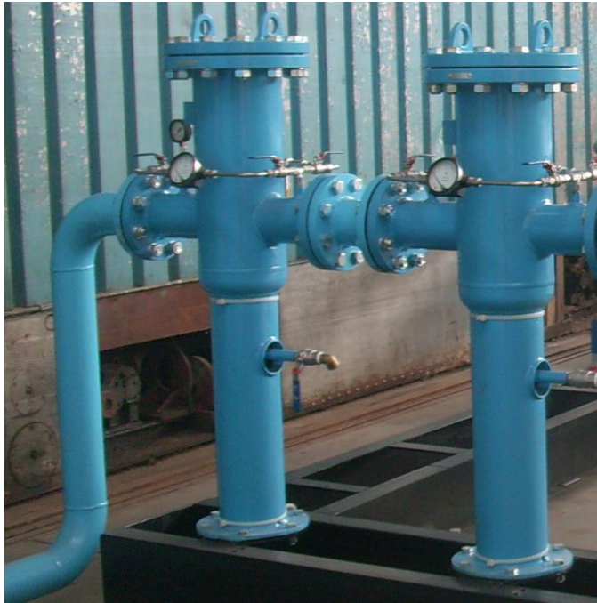
Figure 5. Air conditioning unit – photo of air filtering unit
